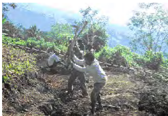
Building a road on top of the mountain. Liquiça District, East Timor © Francis Dobbs, World Bank.
